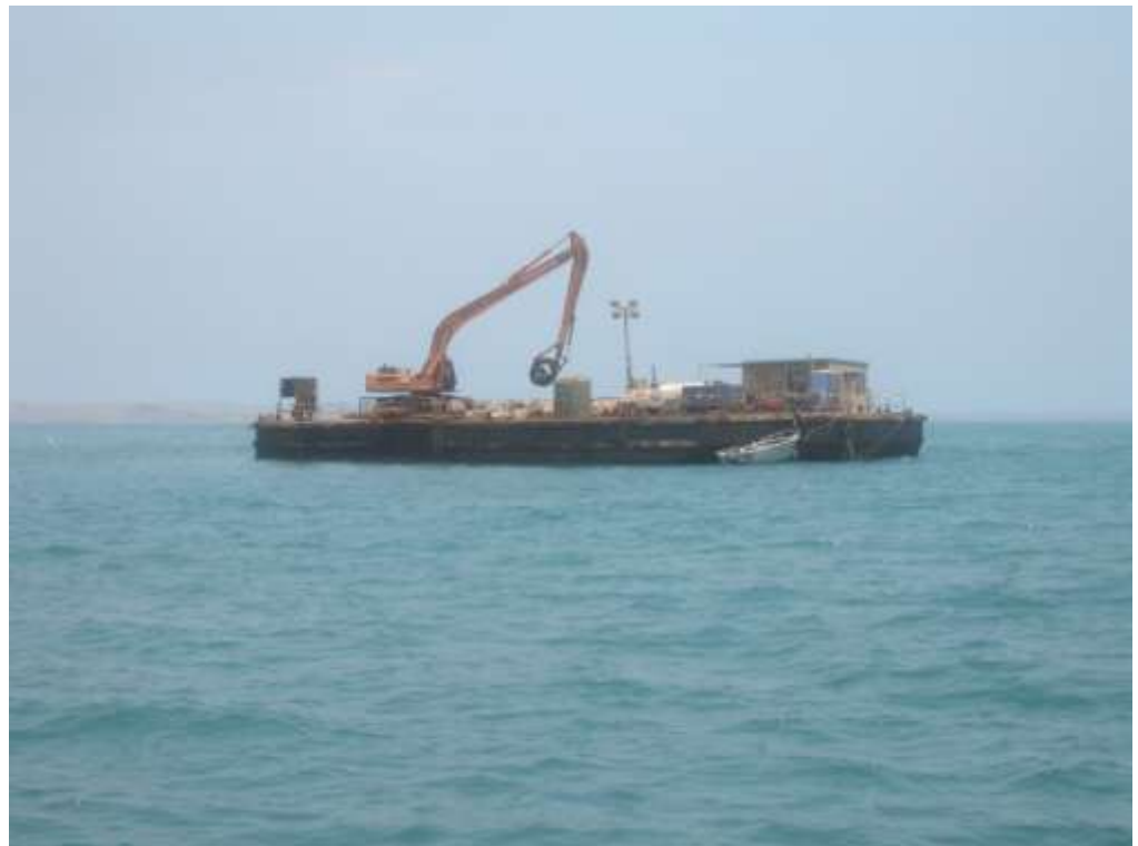
Figure 3. Rock boulders being cleaned in a digger bucket and then craned into place on the Parker Point artificial reef site, December 2006.
